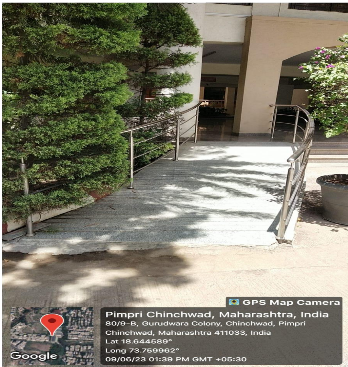
Ramp and rail constructed at the entrance for ease of access to disabled students, staff and visitors
