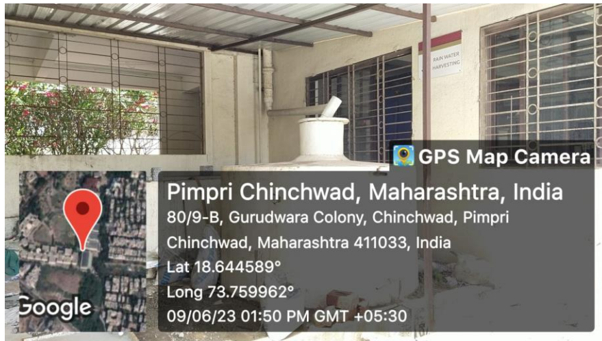
Rain Water Harvesting Plant
