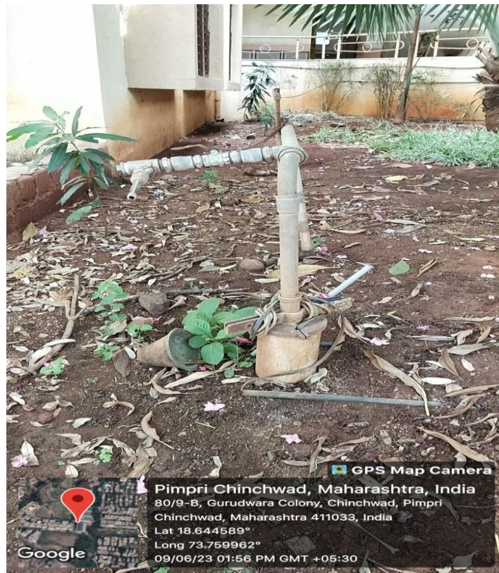
Borewell for digesting rain water
