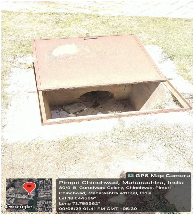
Pits for Rain Water Harvesting
