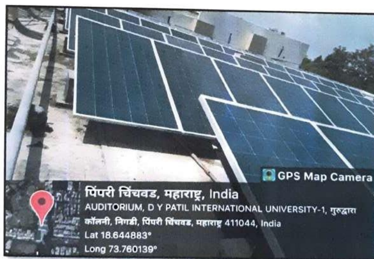
Photograph of Roof Top Solar PV Plant:
