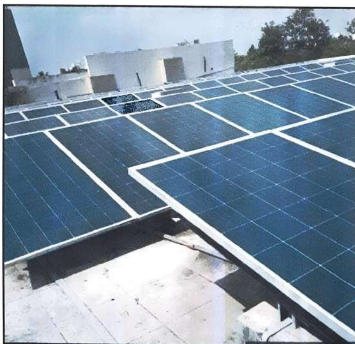
Photograph of Roof Top Solar PV Plant:
