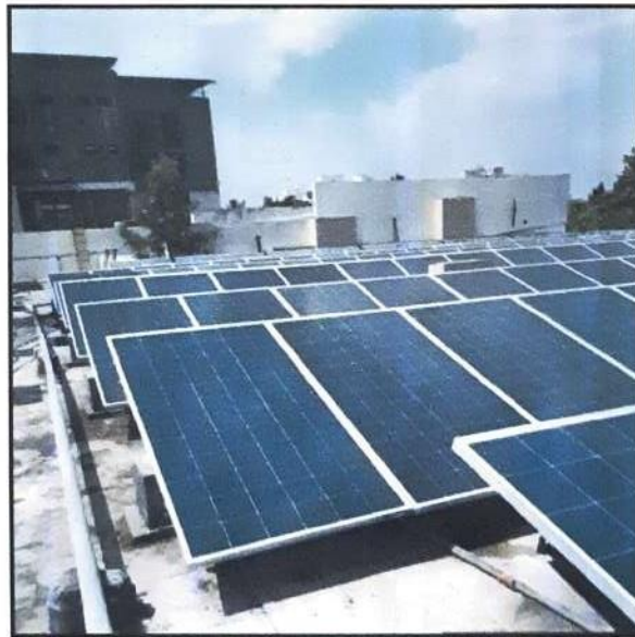
Photograph of Roof Top Solar PV Plant:
