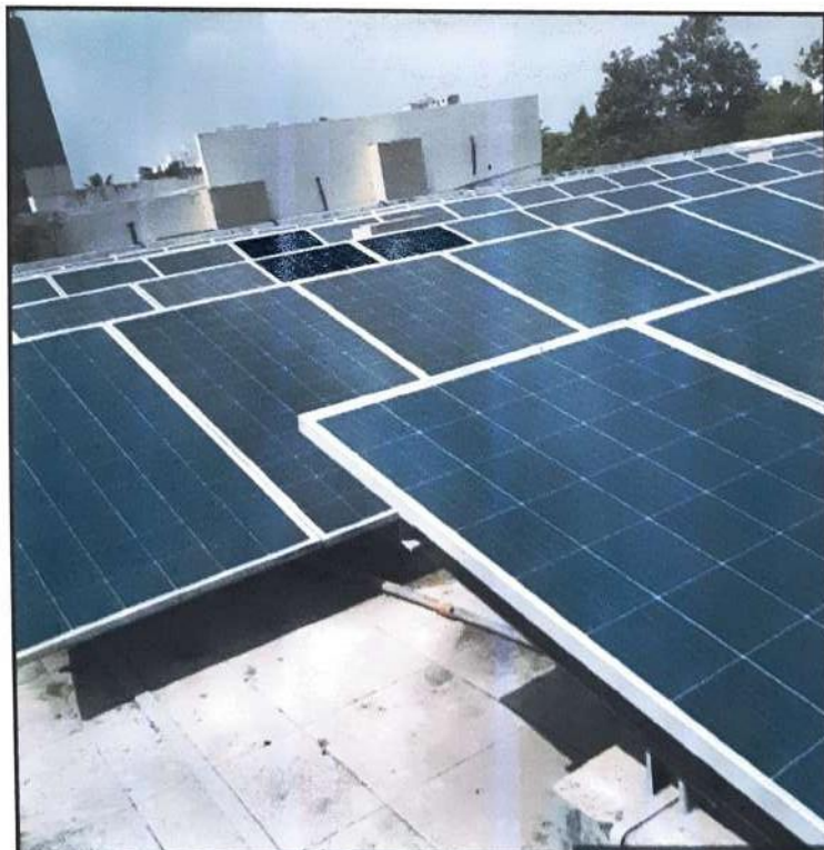
Photograph of Roof Top Solar PV Plant:
