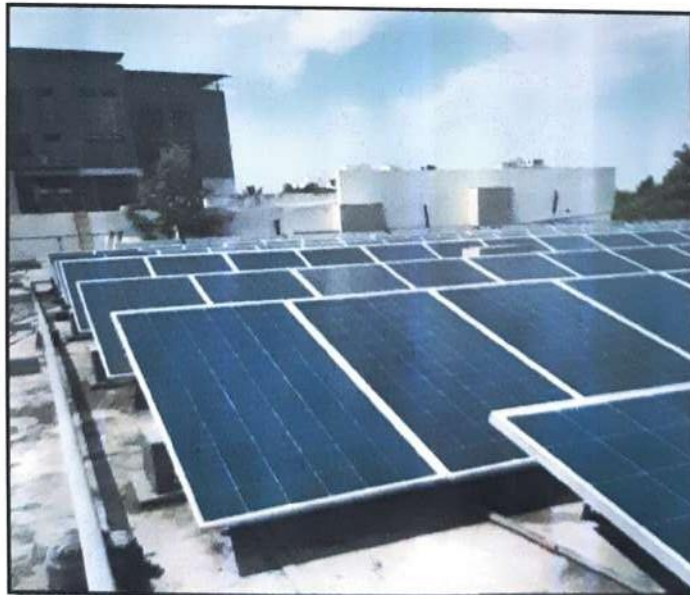
Photograph of Roof Top Solar PV Plant:
