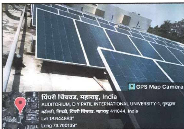
Photograph of Roof Top Solar PV Plant:
