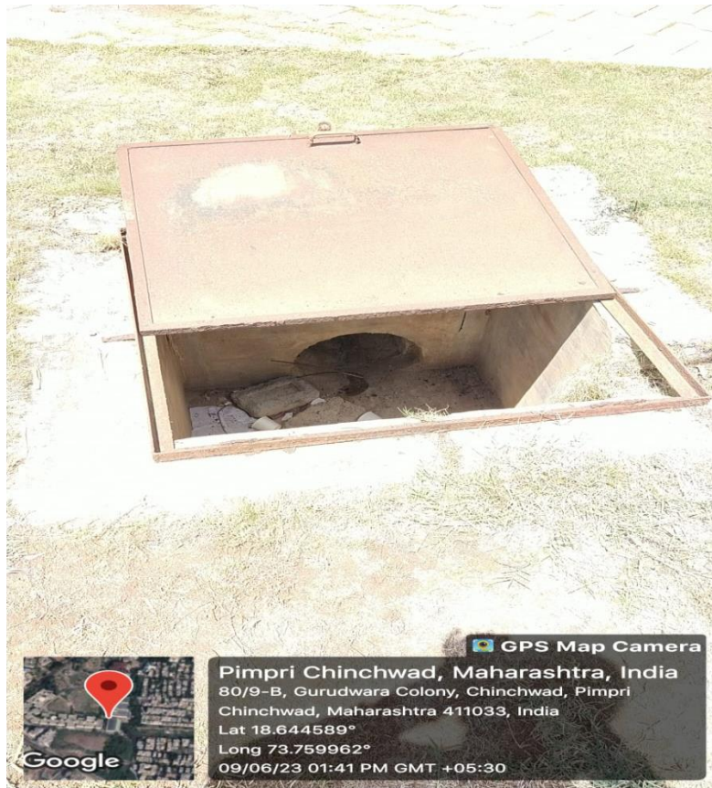
Pits for Rain Water Harvesting
