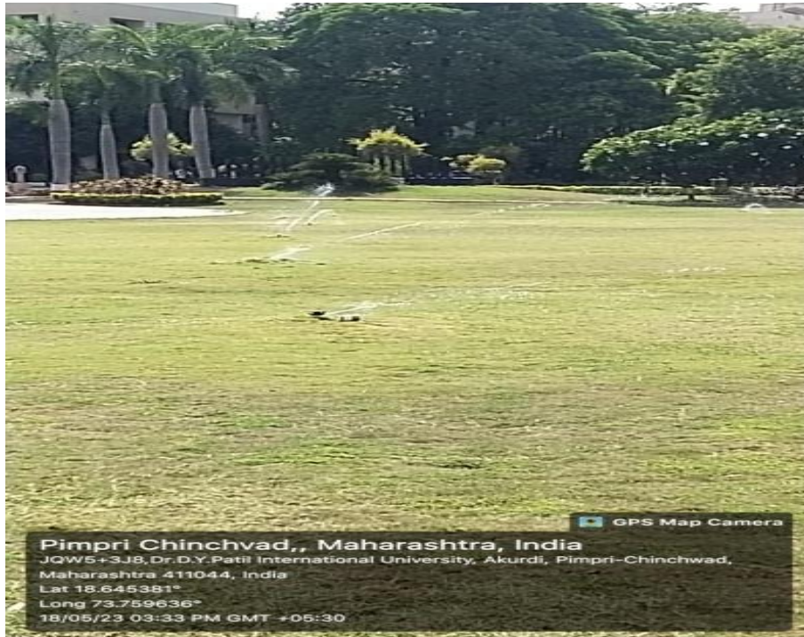
Sprinklers are used for lawn area to save water wastage
